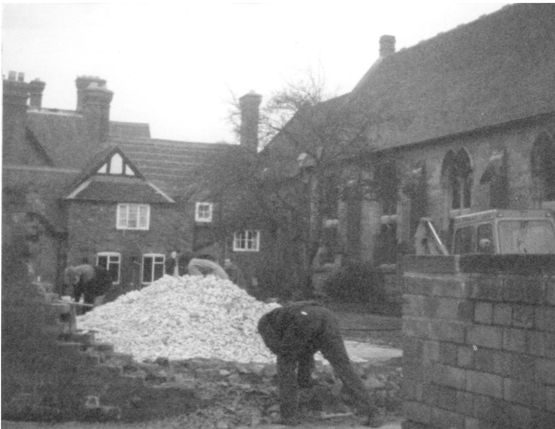
(Work in progress after part of the old vicarage was sold to the Health Authority)
